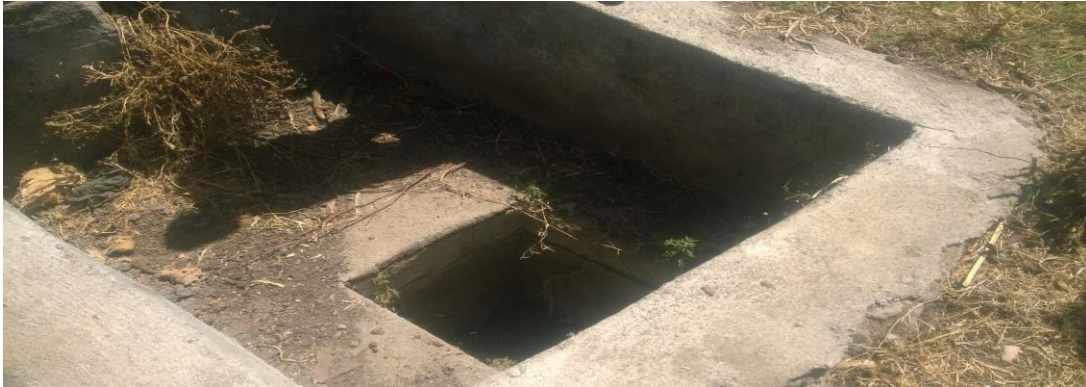
Plate 3 : A fixed dome digester that has been abandoned due to incomplete construction.
