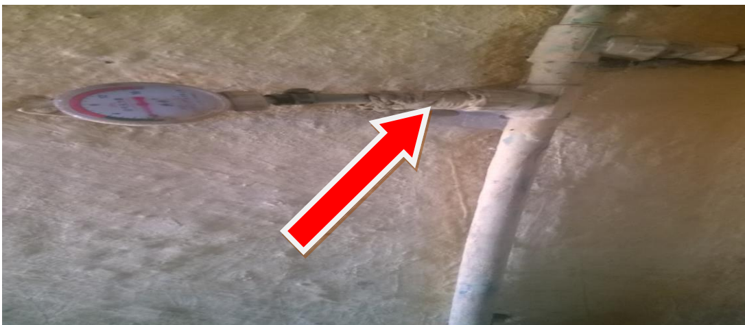
Plate 5: The gas gage which was not connected properly
