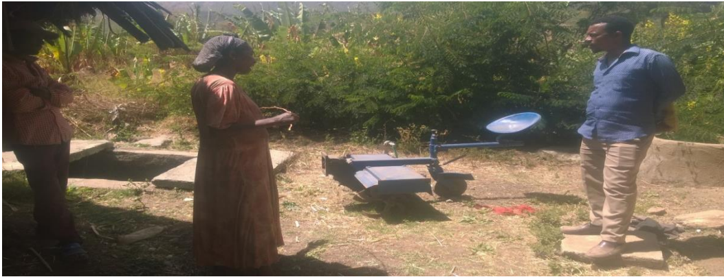
Plate6: Incomplete biogas plants.
