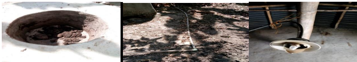
Fig: i ) less or no daily feeding to biogas plant ii ) Installation exposed to gas leakage iii ) Broken glass lamp that are non-functional
