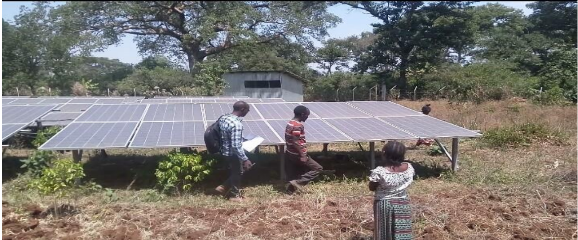
Figure 4.1. Bunata SPV water pumping scheme photo
